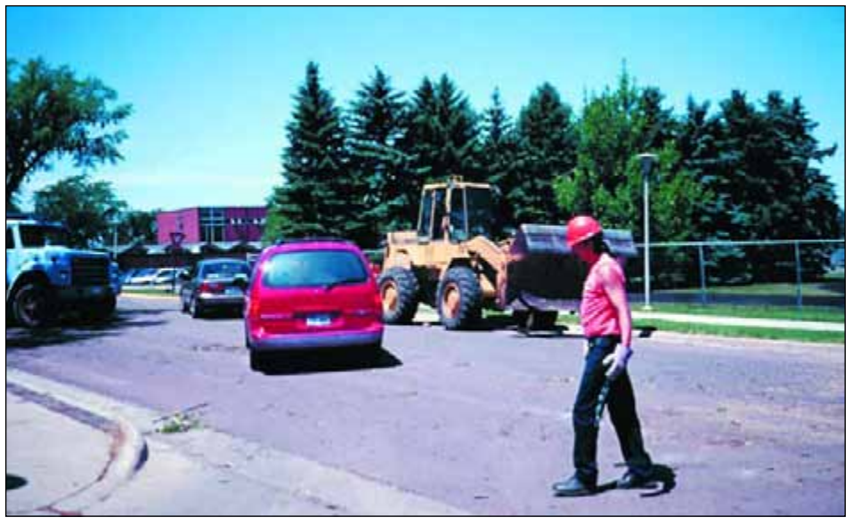
This ground worker just missed being hit by a passing car. The most common on-site transportation fatality is being struck by passing traffic.
